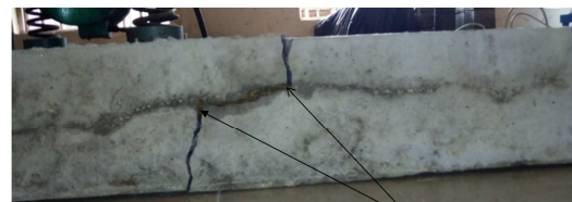
Lines of Fracture
